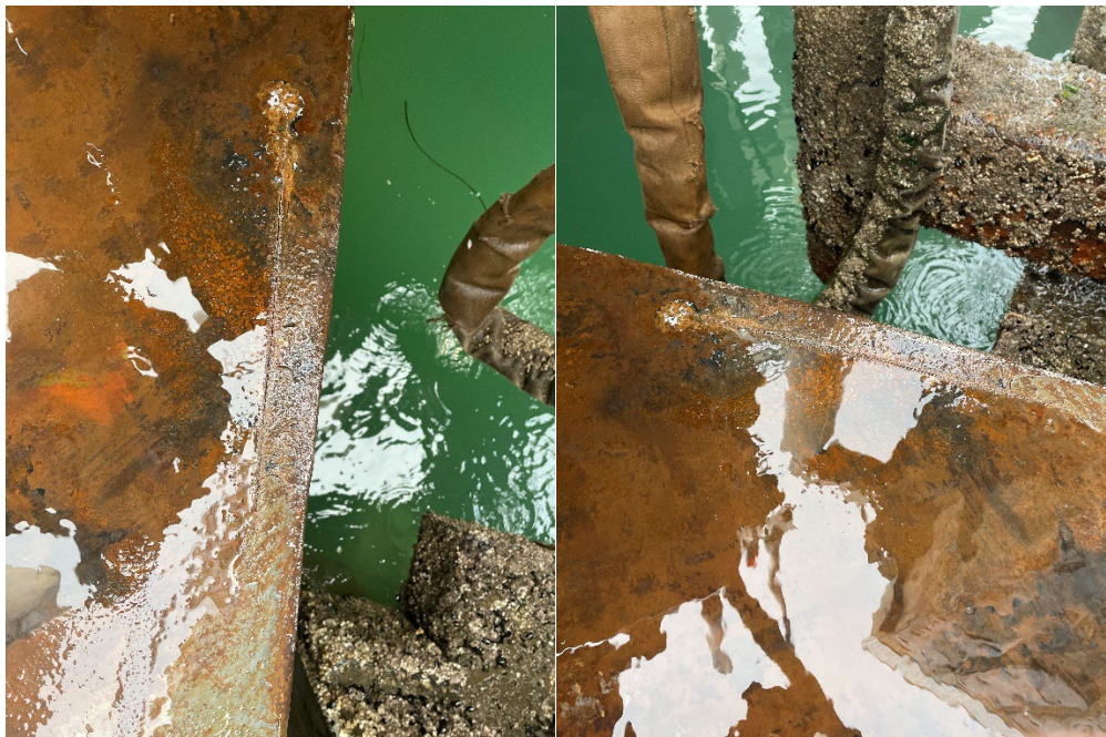
Figure 1 Crack in the Sponson Area
